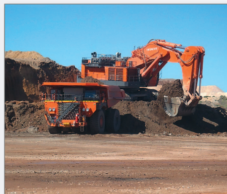
Ultra class equipment being used in a similar method to that proposed for the Hillside Project.
