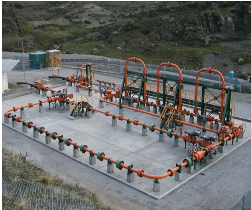
Figure 10 Choke station with vertical choke loops
