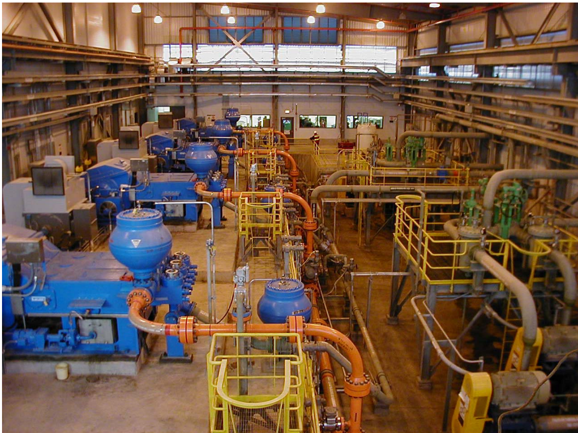
Figure 1 Pump Station PS1
