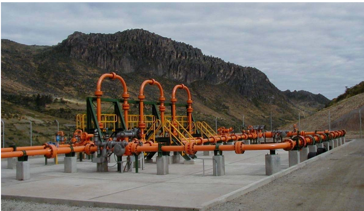
Figure 2 Valve Station 1/Choke Station
