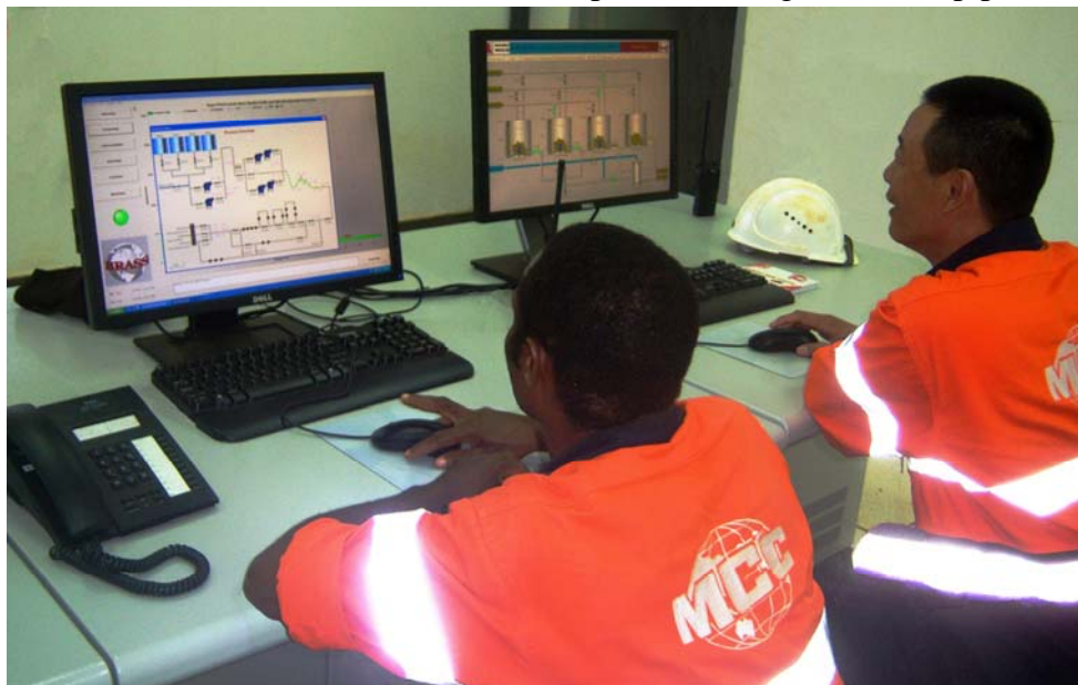
Figure 5 Pipeline Expert™ Control System
